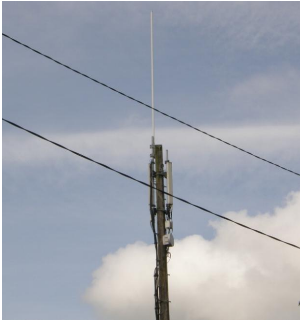
Transmitter Site Photo
